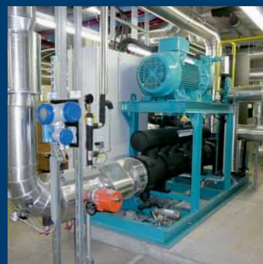
Energy-efficient cooling system in Pottenbrunn (AT)
